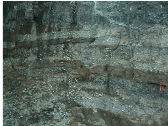
Picture 1.1 Displacement in excavation near Rose Wagner Performing Arts Center.
